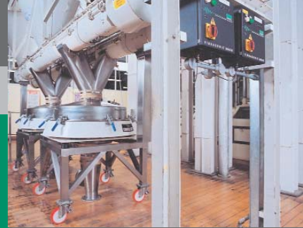
Compact 900 screeners with Vibrasonic debinding system at Colmans - mustard powder producer. The screens are fed from blenders and pass the sieved material through to the packaging area.
