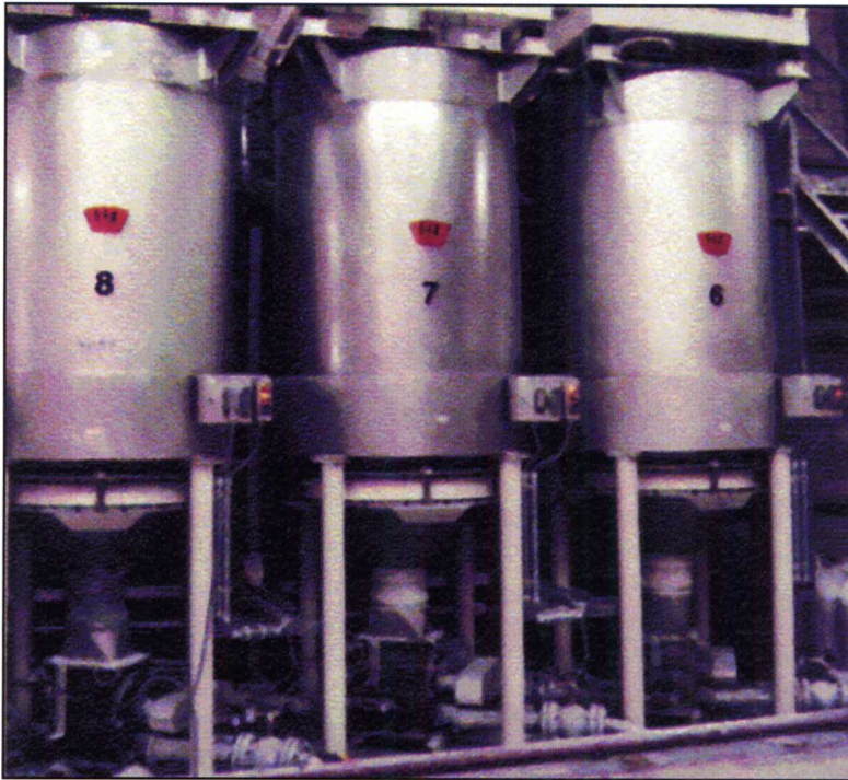
A production line of hoppers with BAV 04 Series Bin Activators.
