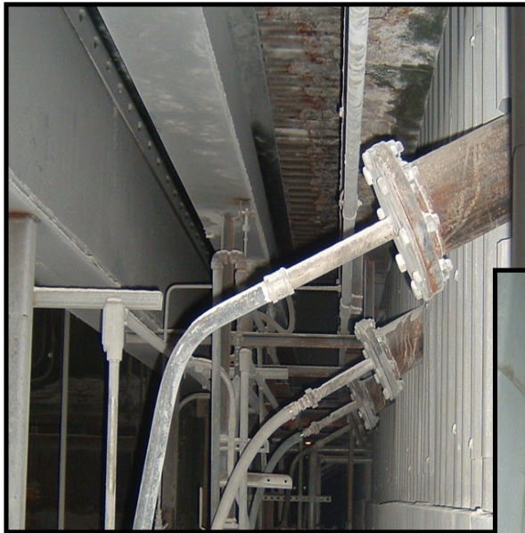
Duct Injection Ports
